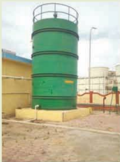
Bio-methanation plant at Sipat
