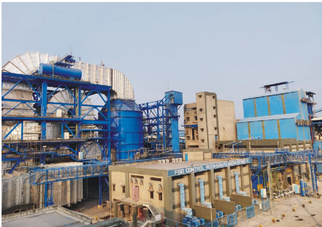
Operational FGD unit, NTPC Vindhyachal
