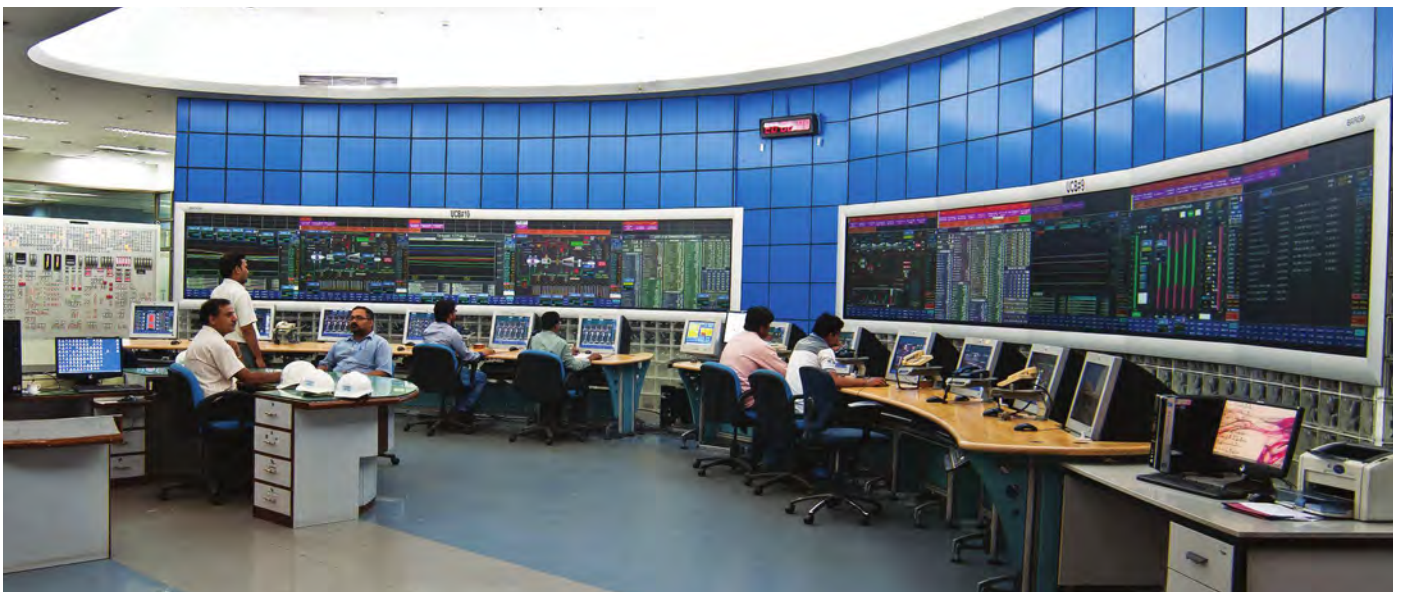
A view of NTPC Control Room
