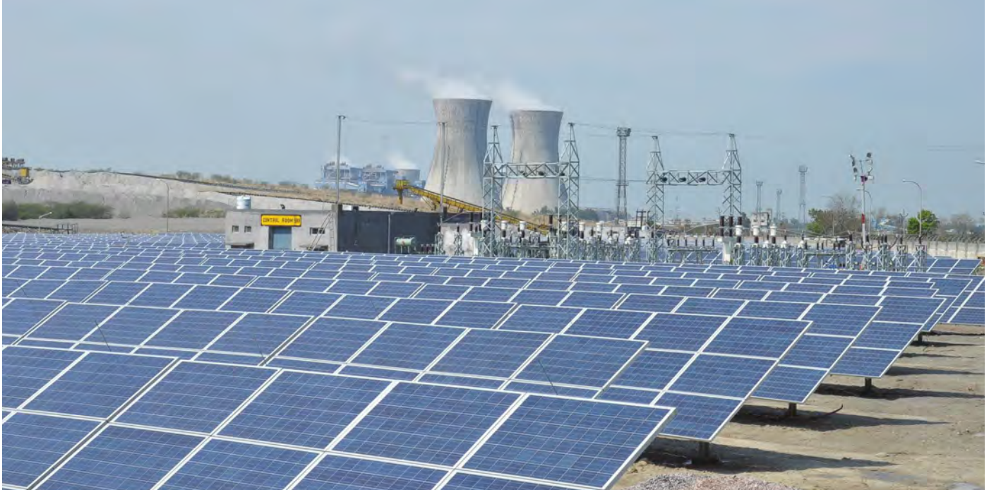
NTPC Dadri Solar Plant
