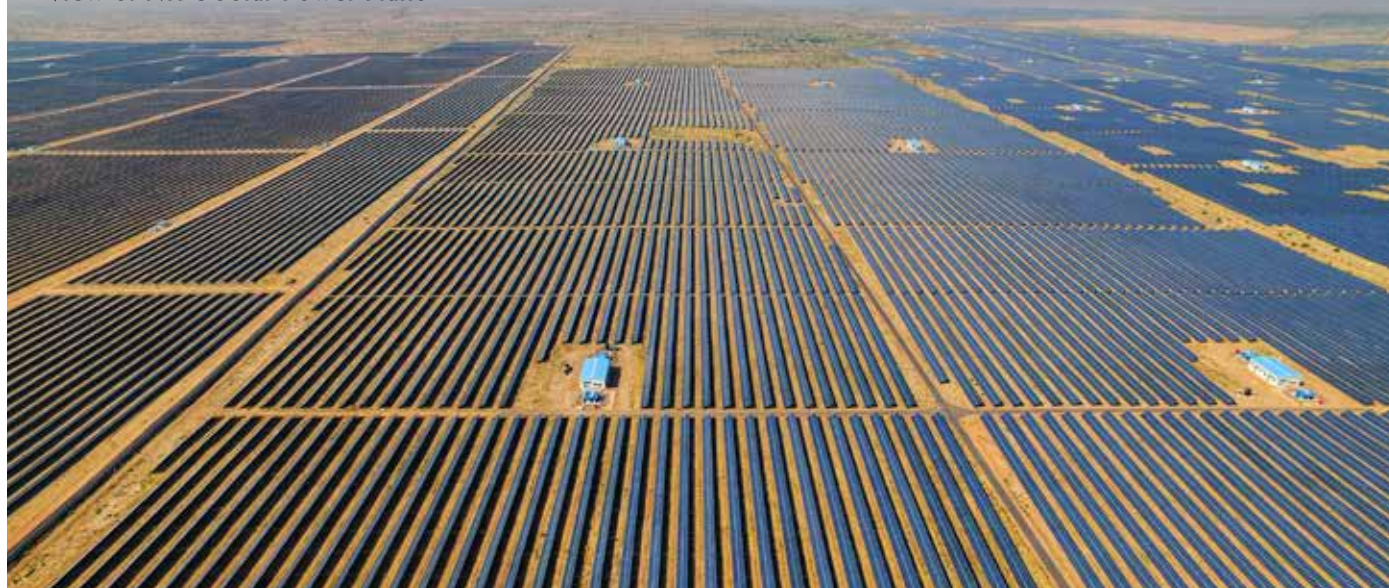
View of NTPC Solar Power Plant
