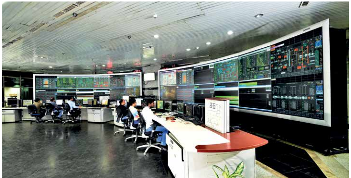
Control Room at NTPC Bongaigaon
