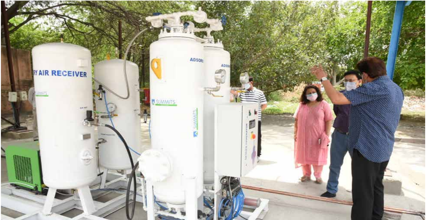
Oxygen Generation Plant installed by NTPC
